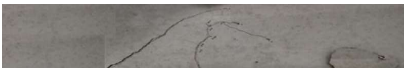
Fig 16: Flexural-shear cracking with concrete crushing – Geopolymer Concrete Sleeper- Mix 3
