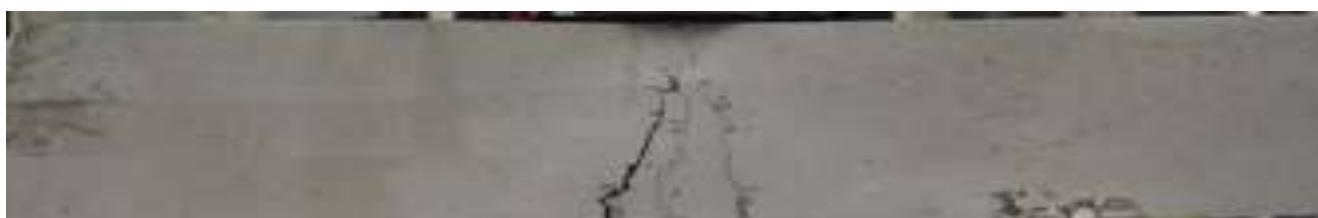
Fig 15: Flexural-shear failure – Geopolymer Concrete Sleeper- Mix 2
