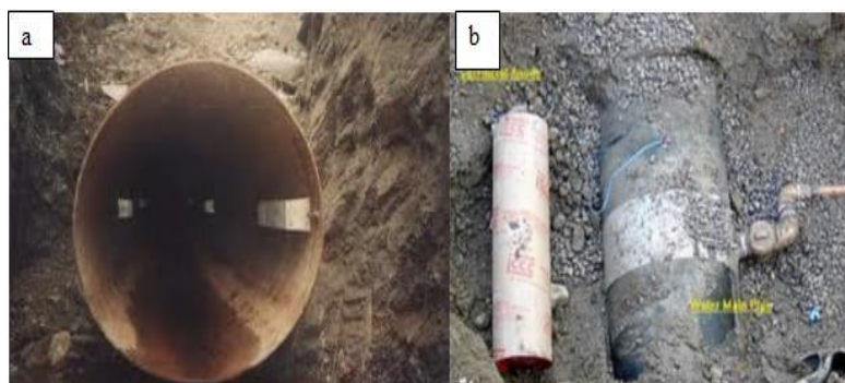
Figure 10. (a) Internal protection of water pipe-line using sacrificial anodic method (b) External protection of water pipe-line using sacrificial anodic method
