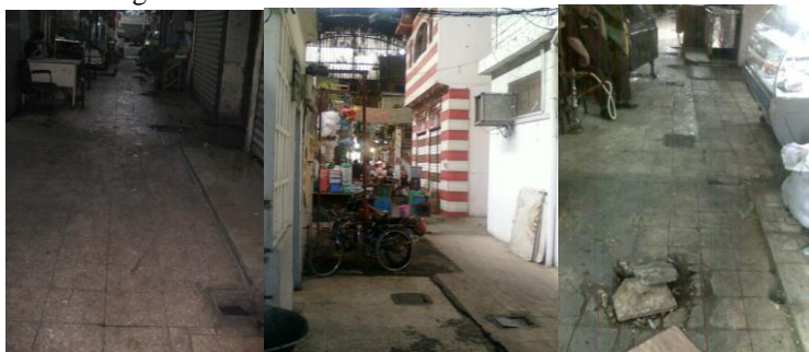
Fig. 14. Deterioration of Floors and Drainage System. Source, Researcher
