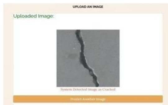
Fig 7: Image Predicted as Cracked
